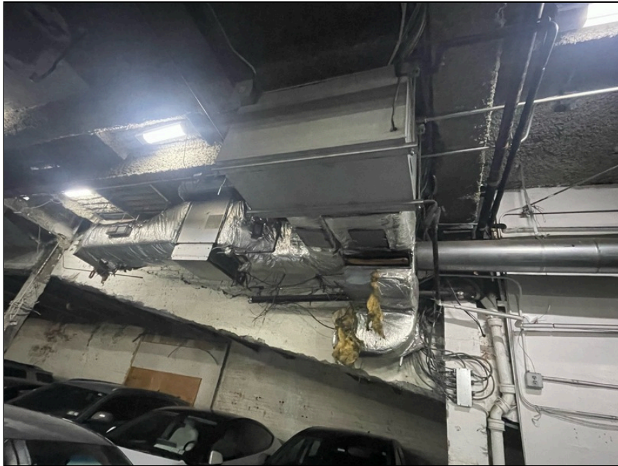
Photo 45: First floor HVAC system
