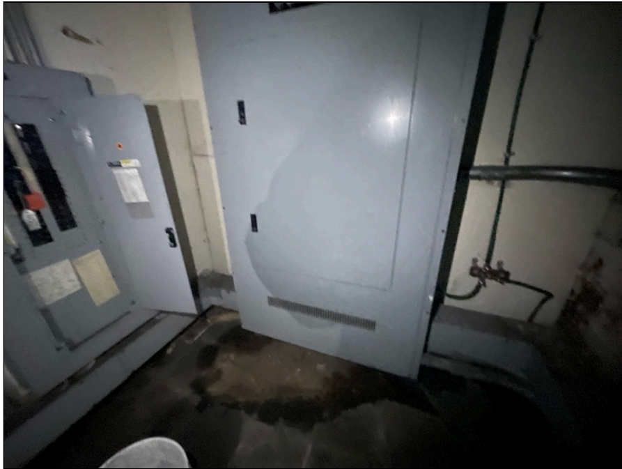
Photo 167: Main electric panels, first floor
