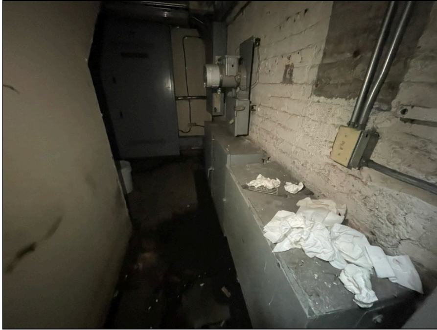
Photo 163: First floor electric room
