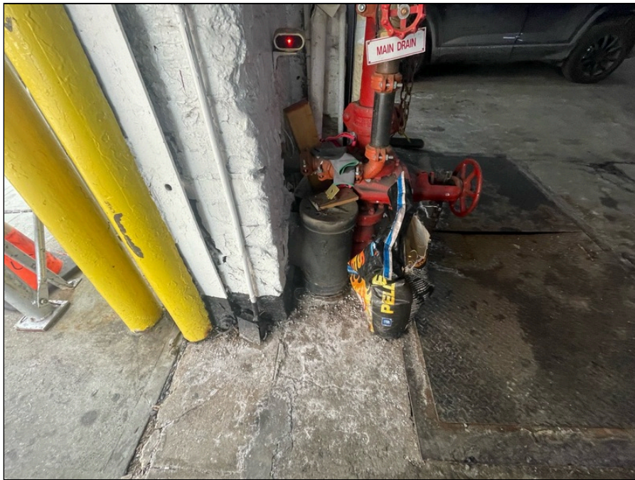
Photo 28: Sprinkler main, first floor
