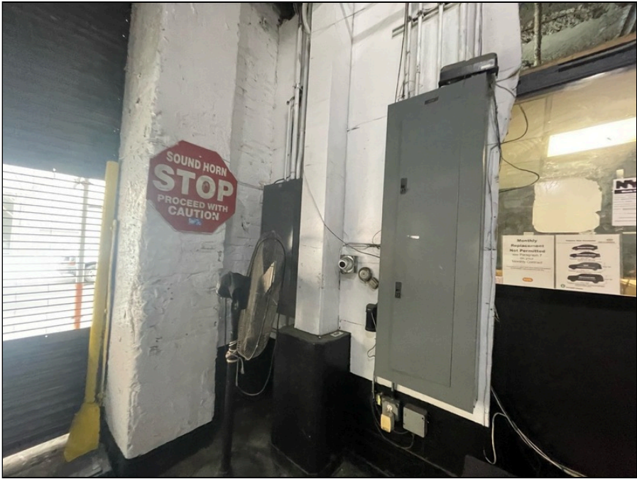
Photo 174: First floor electric panel
