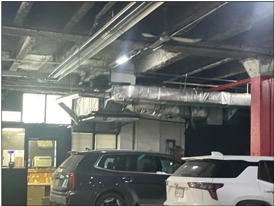
Photo 62: First floor HVAC system
