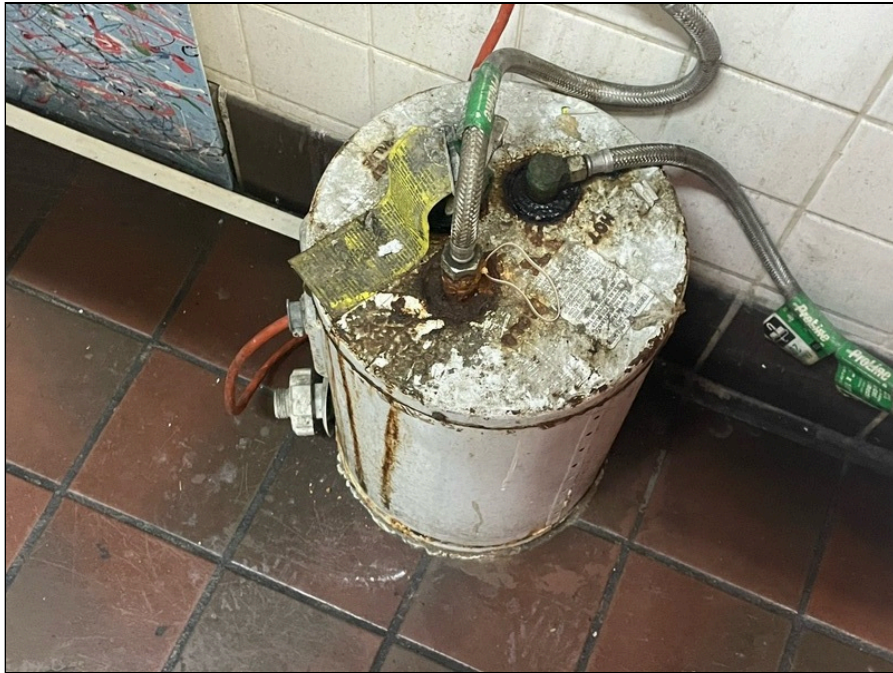
Photo 139: Hot water heaters, second floor
