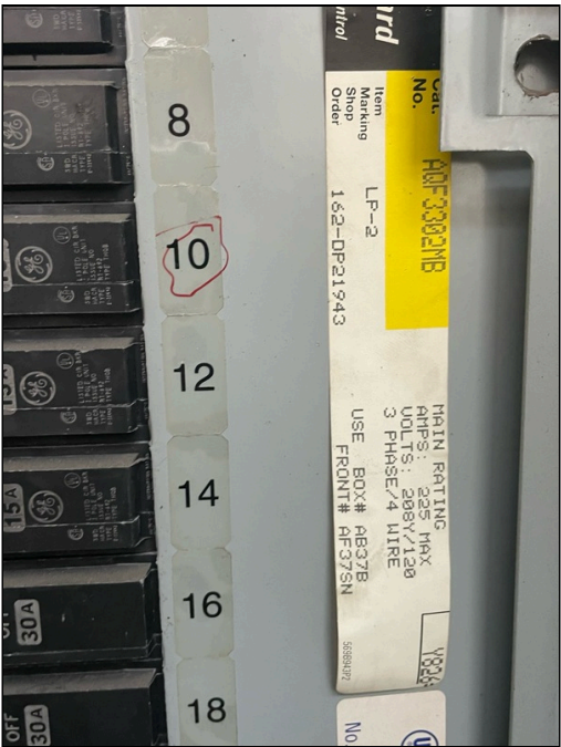
Photo 162: First floor electric panel
