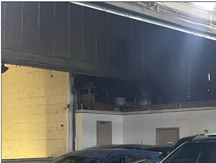
Photo 137: Hot water heaters, second floor
