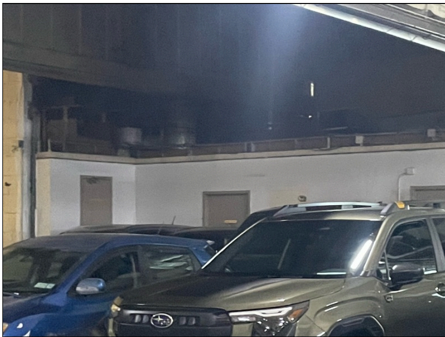
Photo 136: Hot water heaters, second floor
