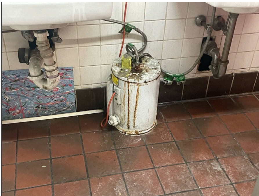
Photo 138: Hot water heaters, second floor
