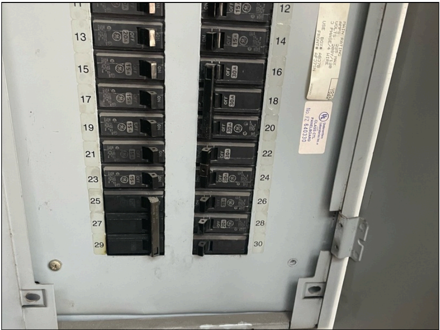
Photo 161: First floor electric panel
