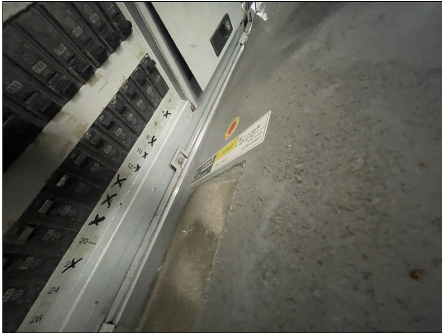
Photo 175: First floor electric panel
