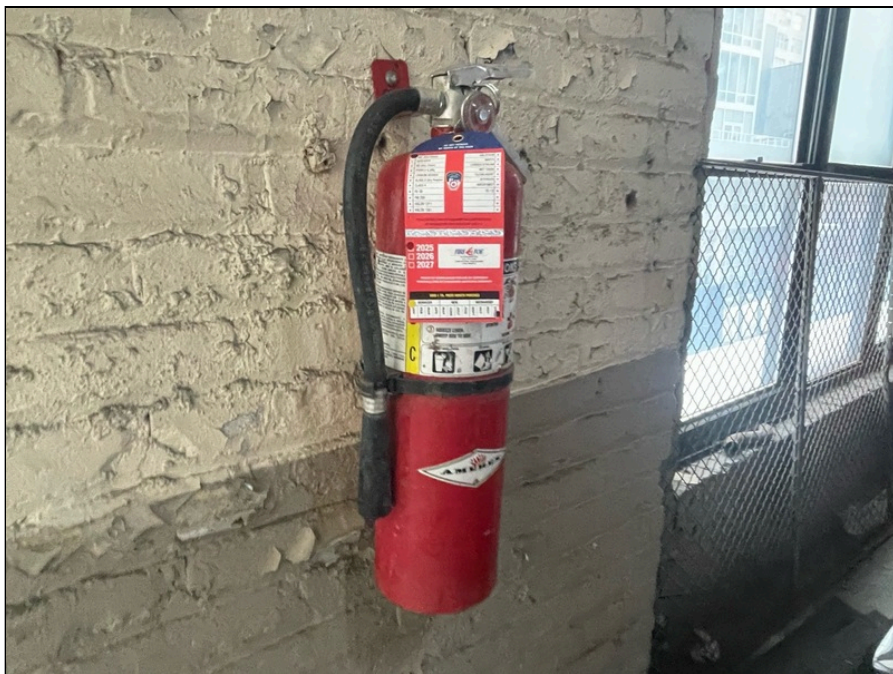
Photo 158: Fire extinguisher, second floor
