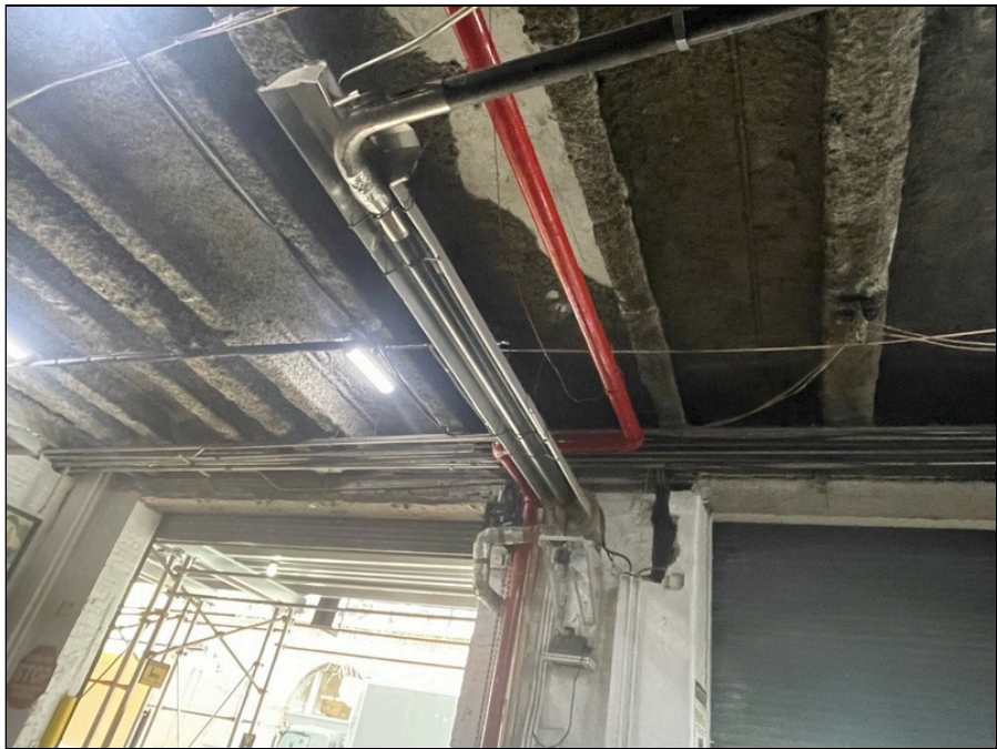
Photo 13: First floor heating system
