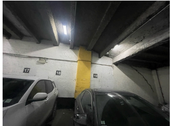
Cracking observed to brick masonry walls
