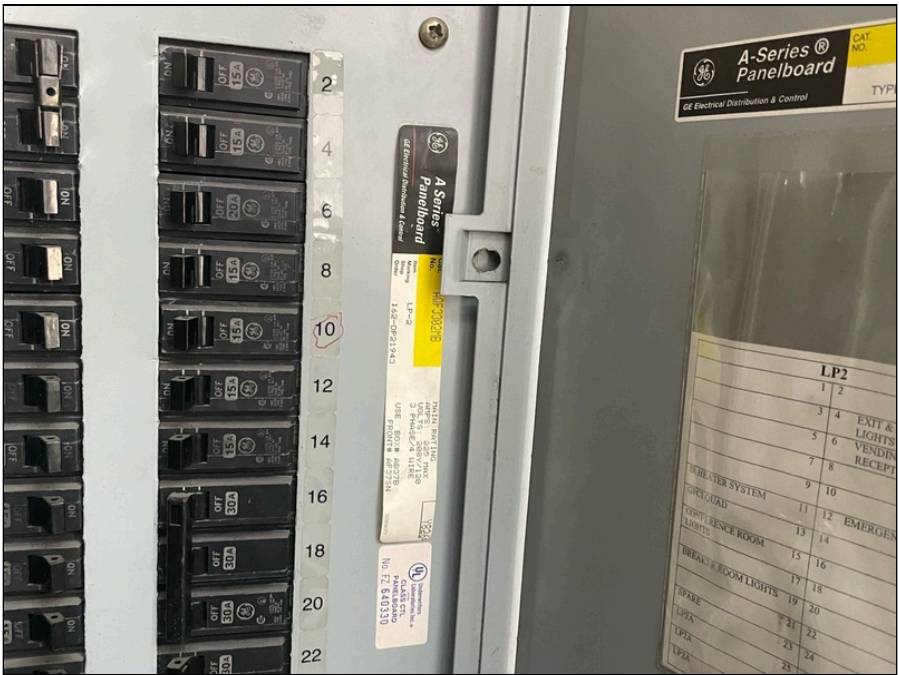
Photo 160: First floor electric panel
