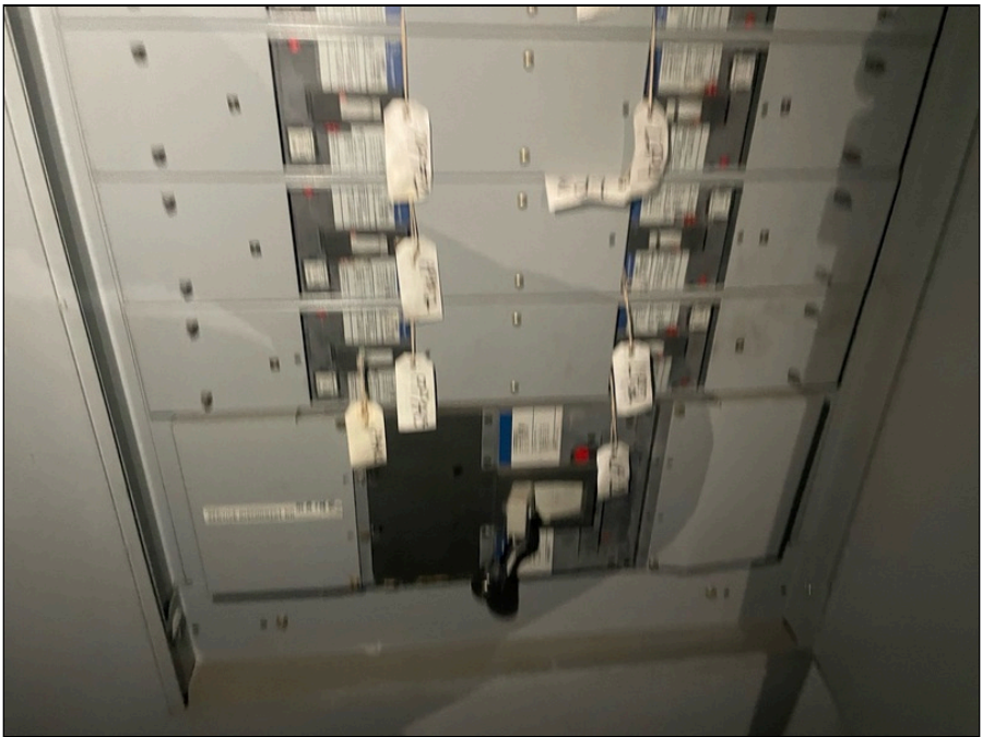
Photo 171: Main electric panels, first floor
