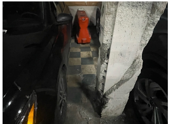
Damaged concrete on support columns
