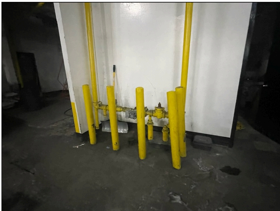
Photo 56: Natural gas meter, first floor
