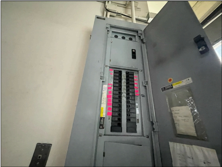
Photo 89: Second floor electric panel
