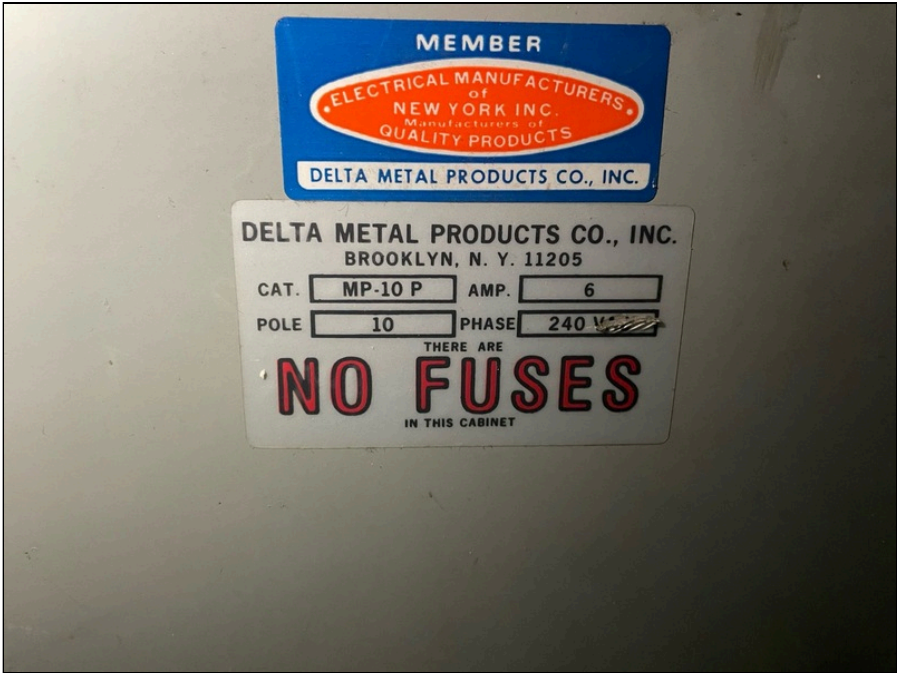
Photo 173: Main electric panels, first floor
