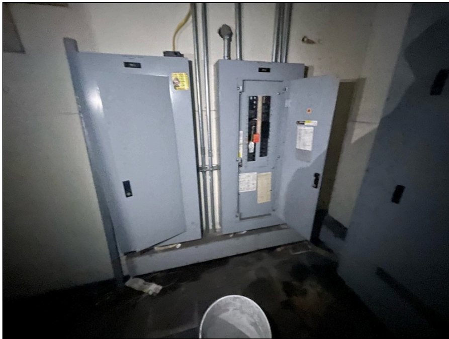
Photo 166: Main electric panels, first floor
