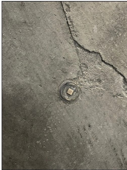
Photo 16: Cleanout, first floor
