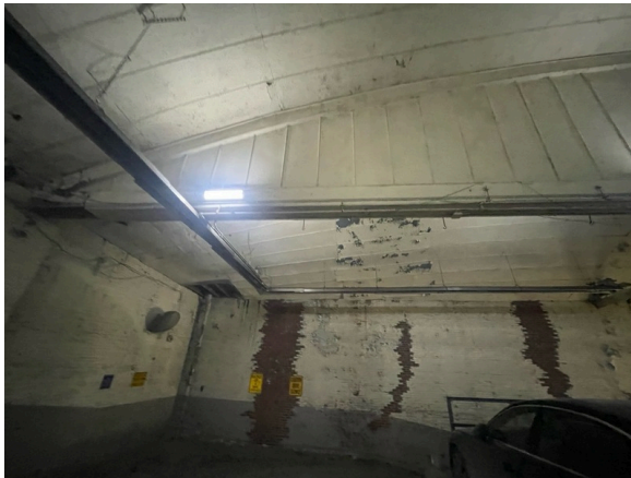
Potentially previous damaged brick masonry
