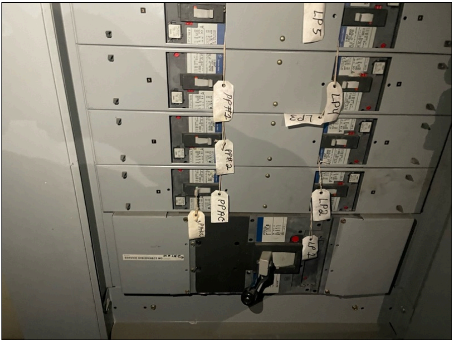
Photo 170: Main electric panels, first floor
