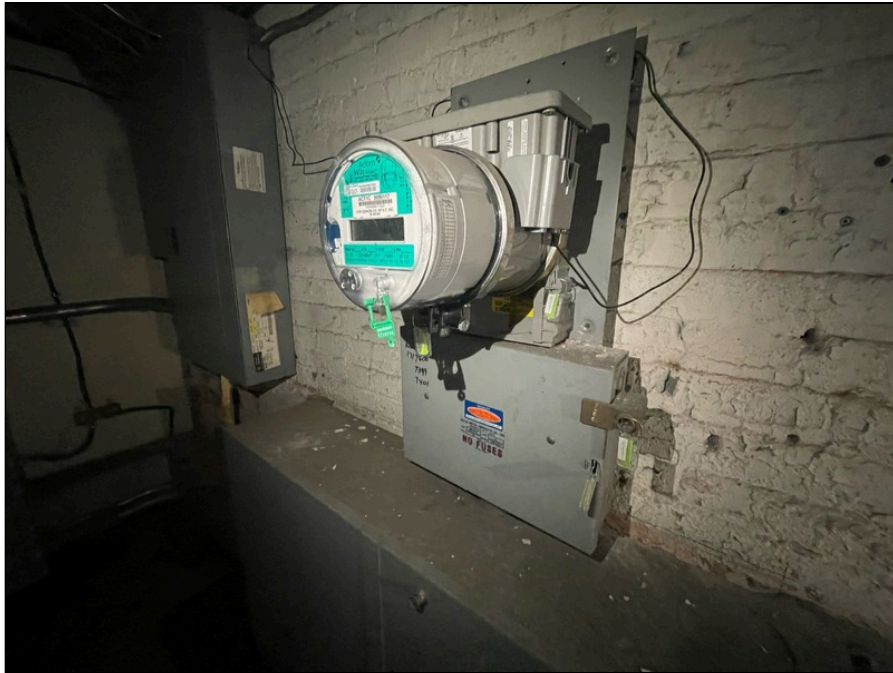
Photo 165: Electric meter, first floor
